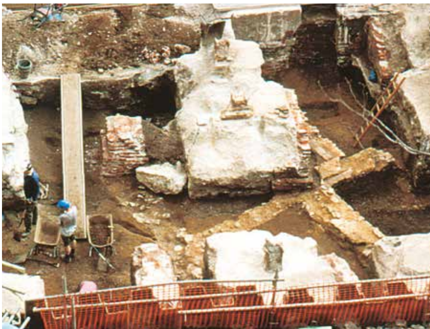
Remains beneath former Haddon House looking south from 68-70 Fenchurch Street. The large white blocks are the foundations of Haddon House, the smaller brick piers are from St. Katherine Coleman church and the walls on a different alignment are Roman.
