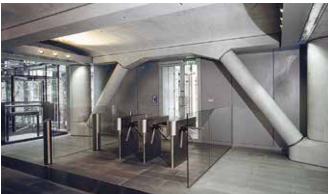
Security turnstiles control movement into the front circulation towers from the entrance hall. The exposed concrete structure plays a part in the building's environmental control. The bottom or top half (as seen here) of the distinctive 'K' bracings can be seen on each floor.
