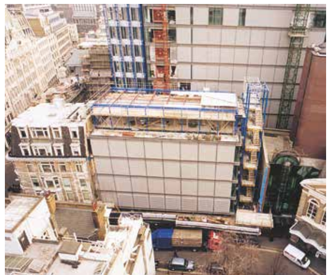
The construction of the Rogers building seen from the west with Fenchurch Street Station on the right – July 1997 and March 1999.
