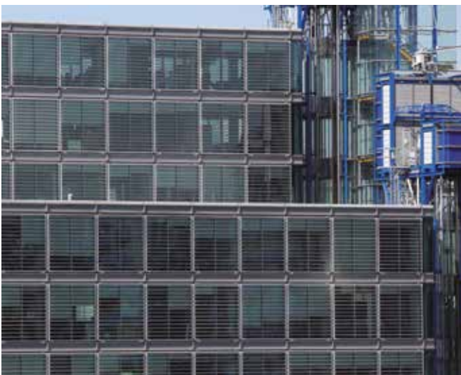
The external louvres on the building's east and west façades are an important means of controlling the office environment.
